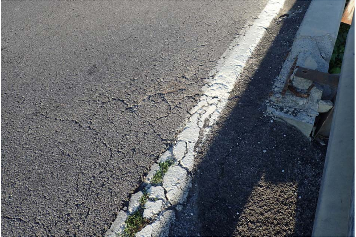
View of rutting and a heavy intensity of cracking along the downstream shoulder of the wearing surface near abutment 2.
