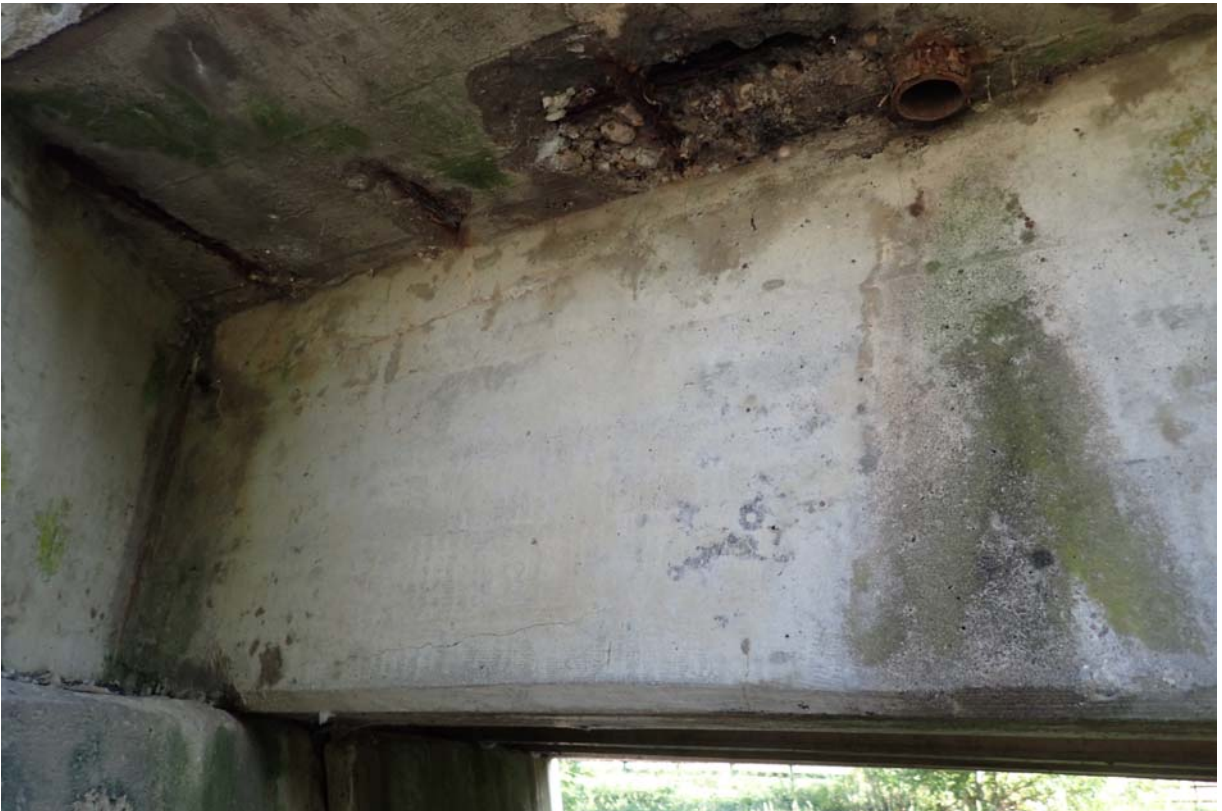
View of minor sized cracking in the upstream beam at abutment 1. Notice the moderate spalling with exposed steel in the deck overhang.
