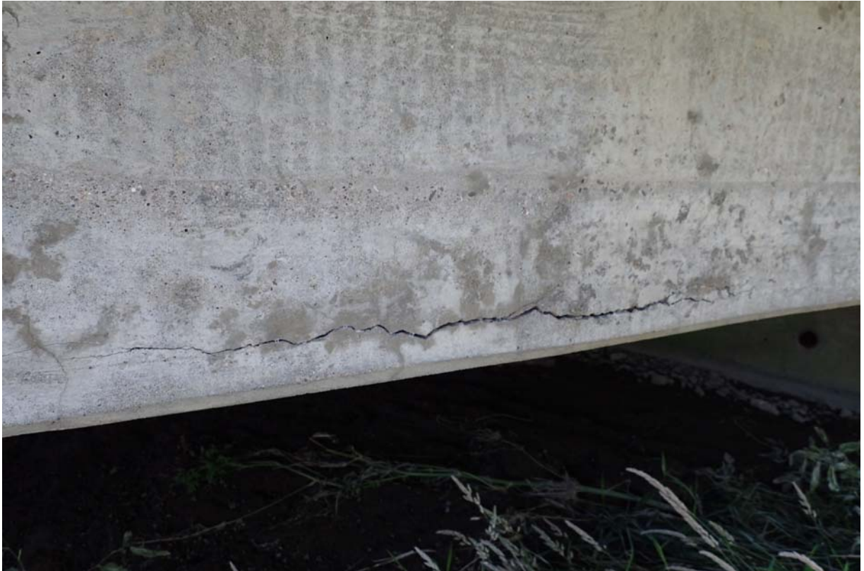
Moderate longitudinal cracking the lower exterior face of the upstream beam near midspan.
