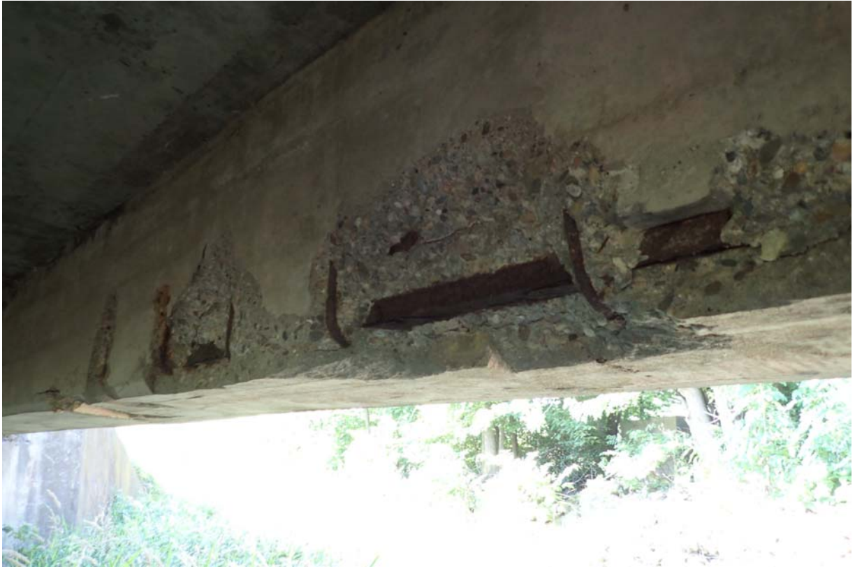
View of heavy spalling with exposed steel in the interior face of the upstream beam near midspan. Notice the exposed longitudinal reinforcement.
