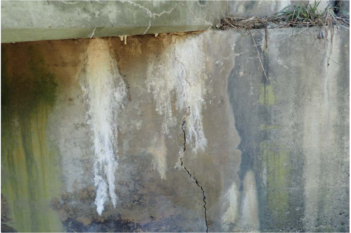
View of a 3/16" wide vertical crack in abutment 2 below the upstream beam.
