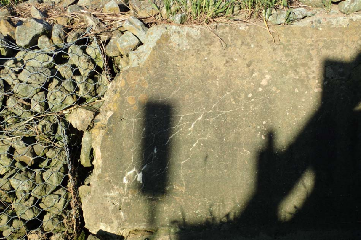
View of moderate spalling and minor sized cracking at the upstream end of abutment 1s wingwall.
