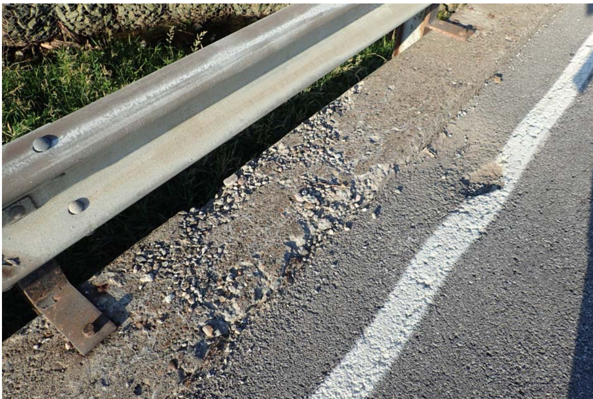
View of moderate spalling in the upstream curb near abutment 2.
