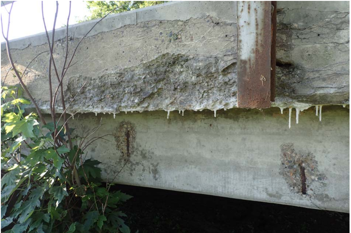
View of heavy spalling in the downstream deck overhang near guardrail post 4 from the south. Notice the moderate spalls with exposed steel in the beam.
