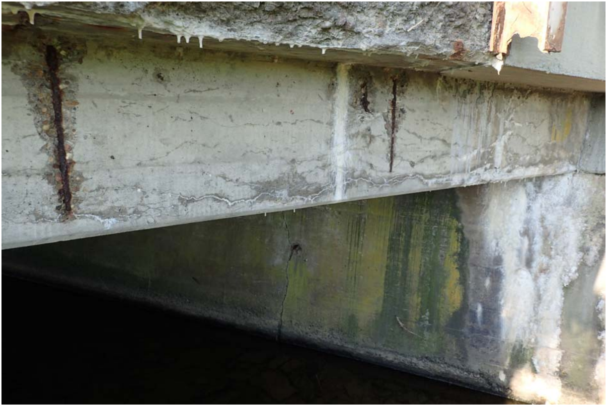
View of minor sized cracking of moderate-heavy intensity in the exterior face of the downstream beam near abutment 1. Notice the shallow spalling with exposed steel in the beam.
