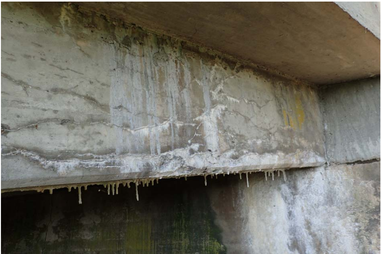
View of minor sized cracking of moderate-heavy intensity in the exterior face of the downstream beam near abutment 1.
