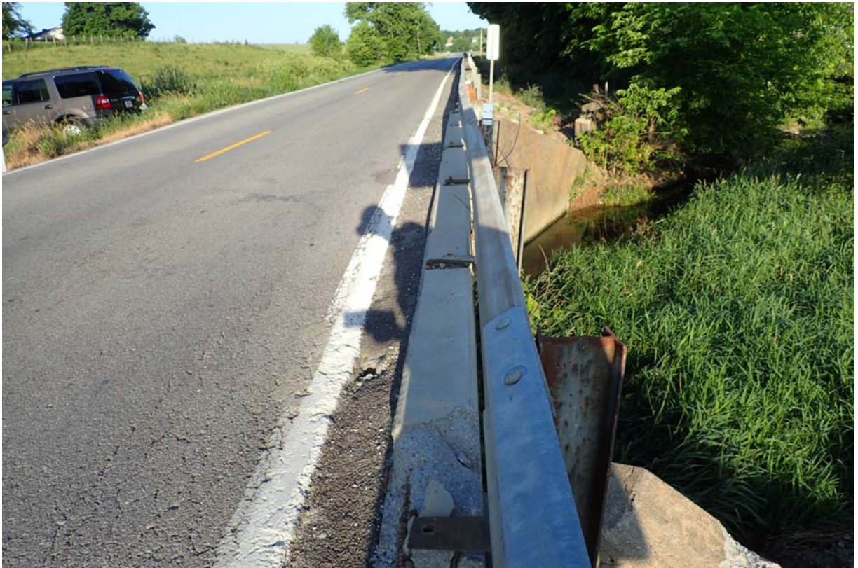
View of the downstream guardrail pushed out from the bridge.
