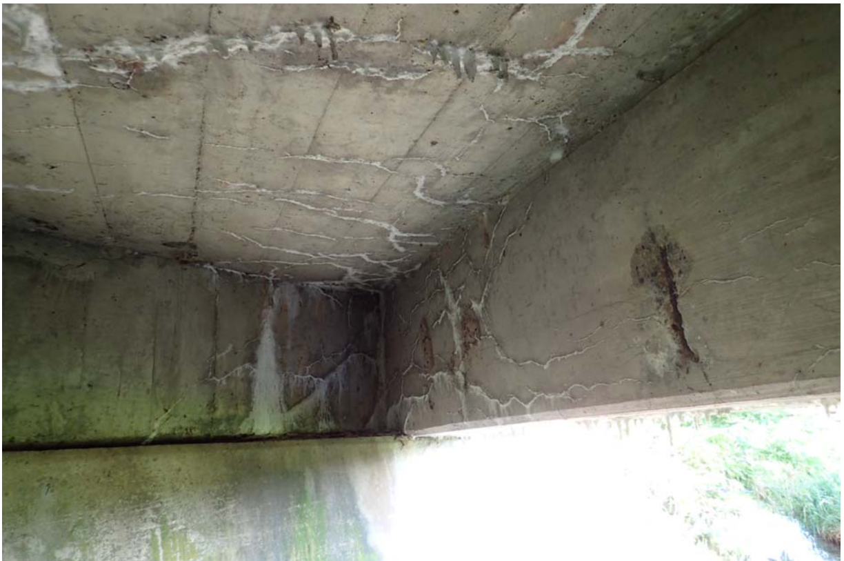
View of a heavy intensity of minor sized cracking with efflorescence in the deck, downstream beam, and diaphragm at/near abutment 1.
