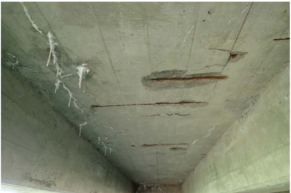
View of scattered cracking with efflorescence and spalling with exposed steel in the deck underside between beams 3 and 4 from upstream.
