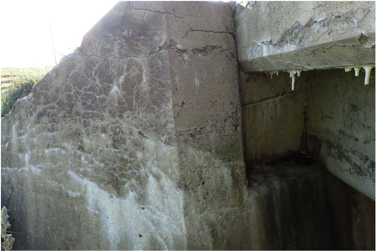
View of minor to moderate sized cracking (heavy intensity) at the downstream end of abutment 2.
