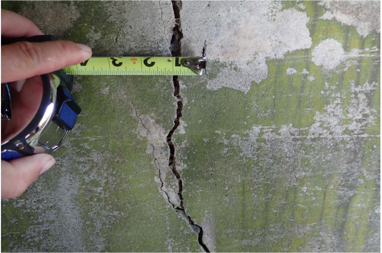
View of a 3/16" wide (typically) crack in abutment 1 below beam 3 from upstream.
