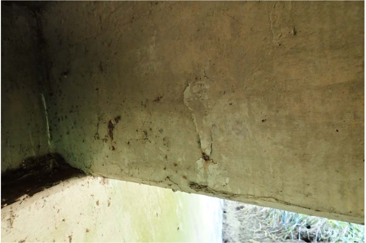
View of minor delamination cracking in the downstream face of beam 2 from upstream near abutment 2.
