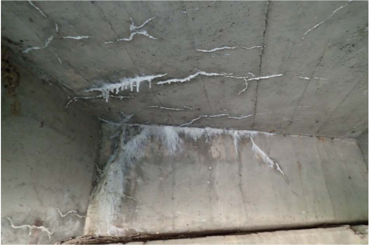
View of moderate to heavy intensity of minor sized cracking with efflorescence in the deck underside and diaphragm between beams 3 and 4 from upstream at abutment 2.
