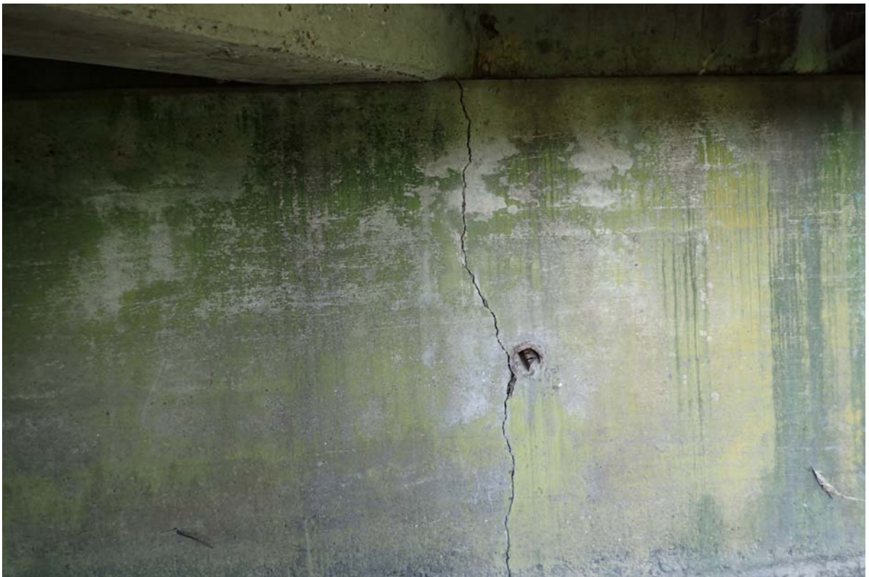
View of a 3/16" wide (typically) crack in abutment 1 below beam 3 from upstream.
