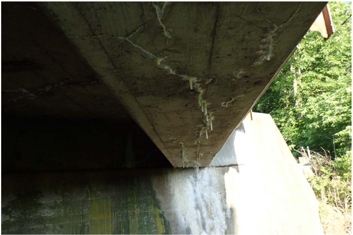
View of cracking with efflorescence in the underside of the downstream beam near abutment 1.
