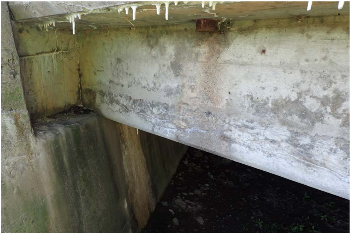
View of minor sized cracking of moderate intensity in the exterior face of the downstream beam near abutment 2.
