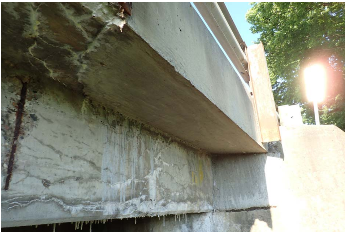
View of a patched area in the downstream overhang near abutment 1.
