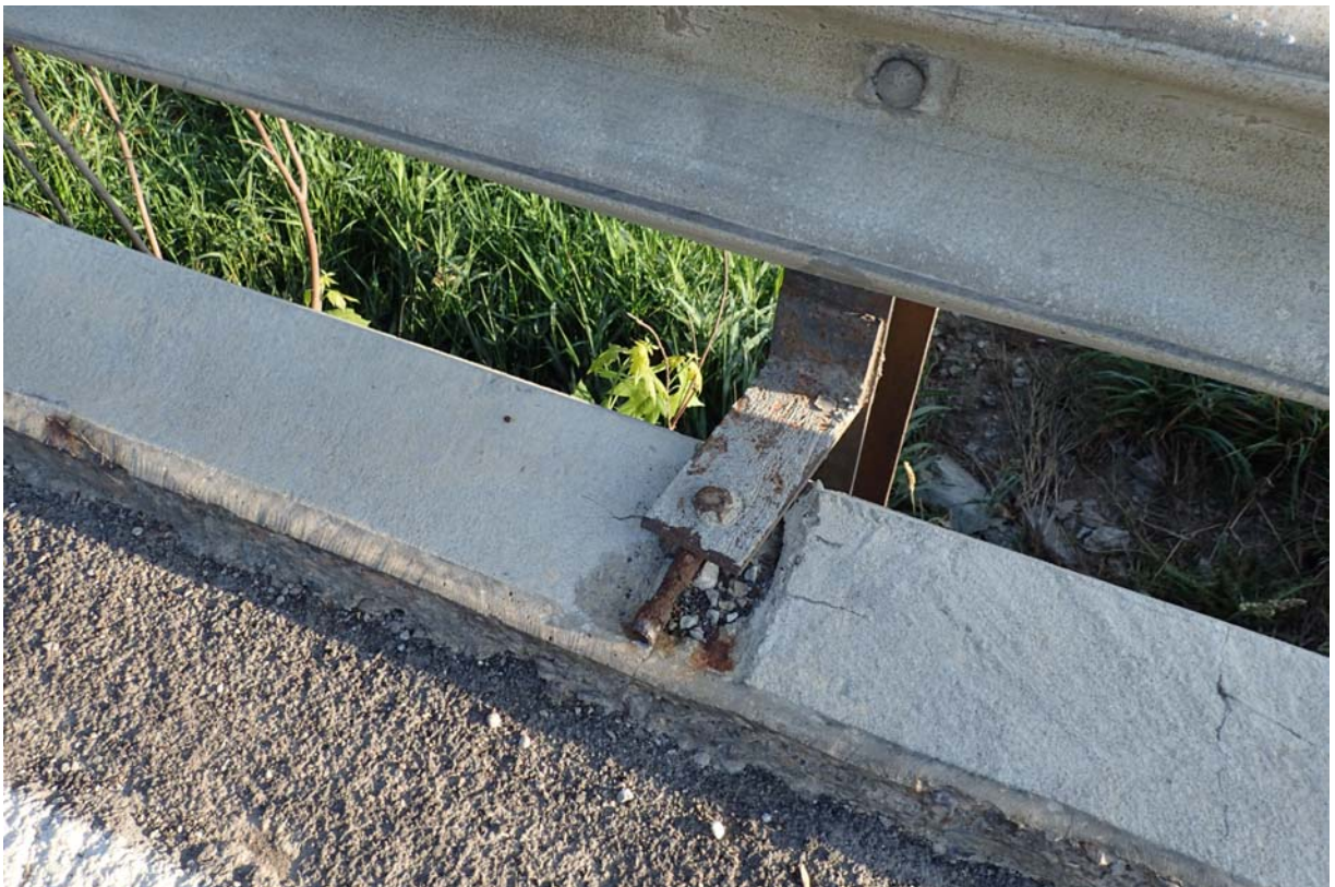
View of disconnected guardrail post 2 from the north in the downstream curb.
