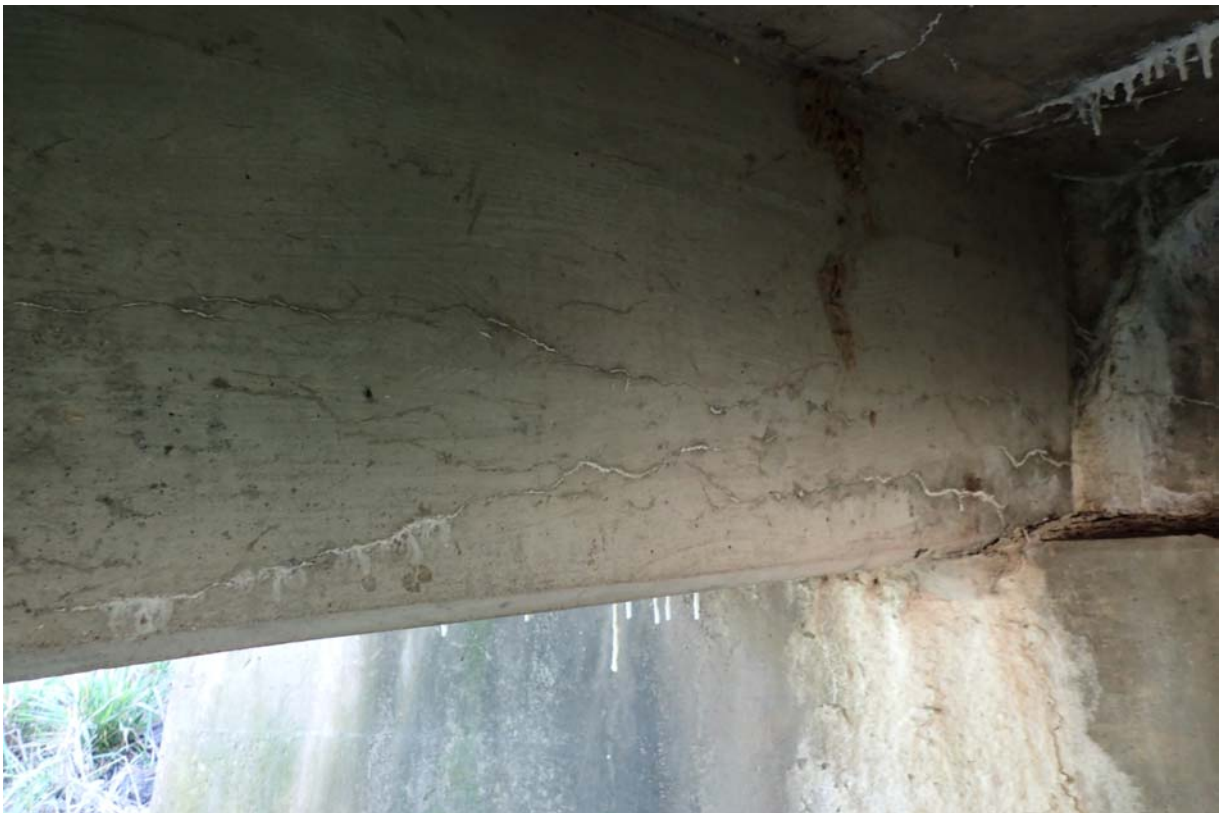
View of minor sized cracking of moderate intensity in the interior face of the downstream beam near abutment 2.
