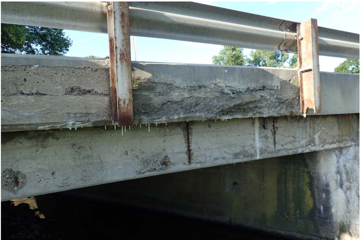
View of heavy spalling in the downstream deck overhang between guardrail posts 2 and 3 from the south. Notice the moderate spalls with exposed steel in the beam.
