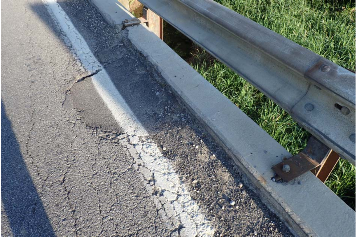
View of rutting, patching, and a heavy intensity of cracking along the downstream shoulder of the wearing surface.
