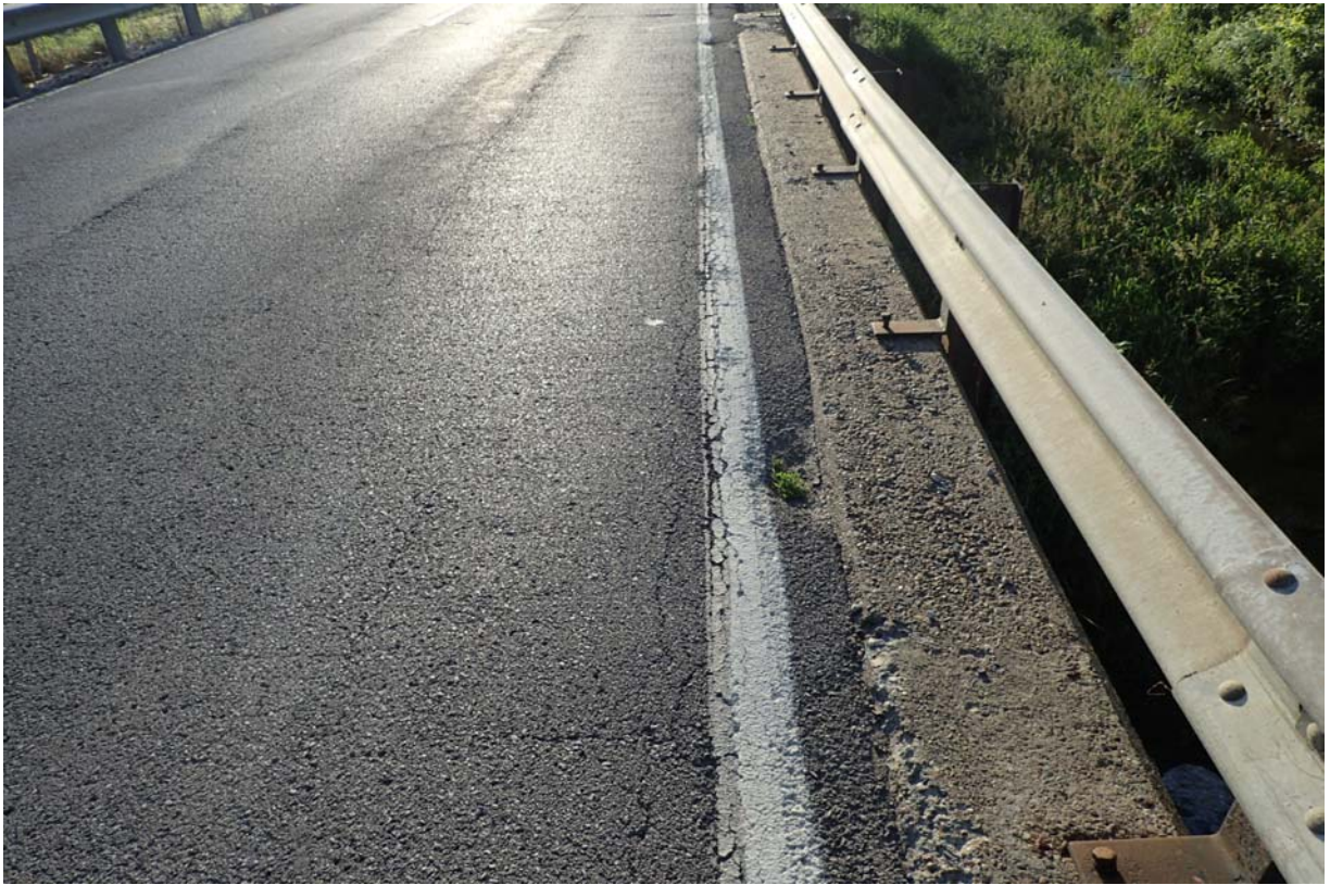
View of minor to moderate scaling/spalling along the downstream curb.
