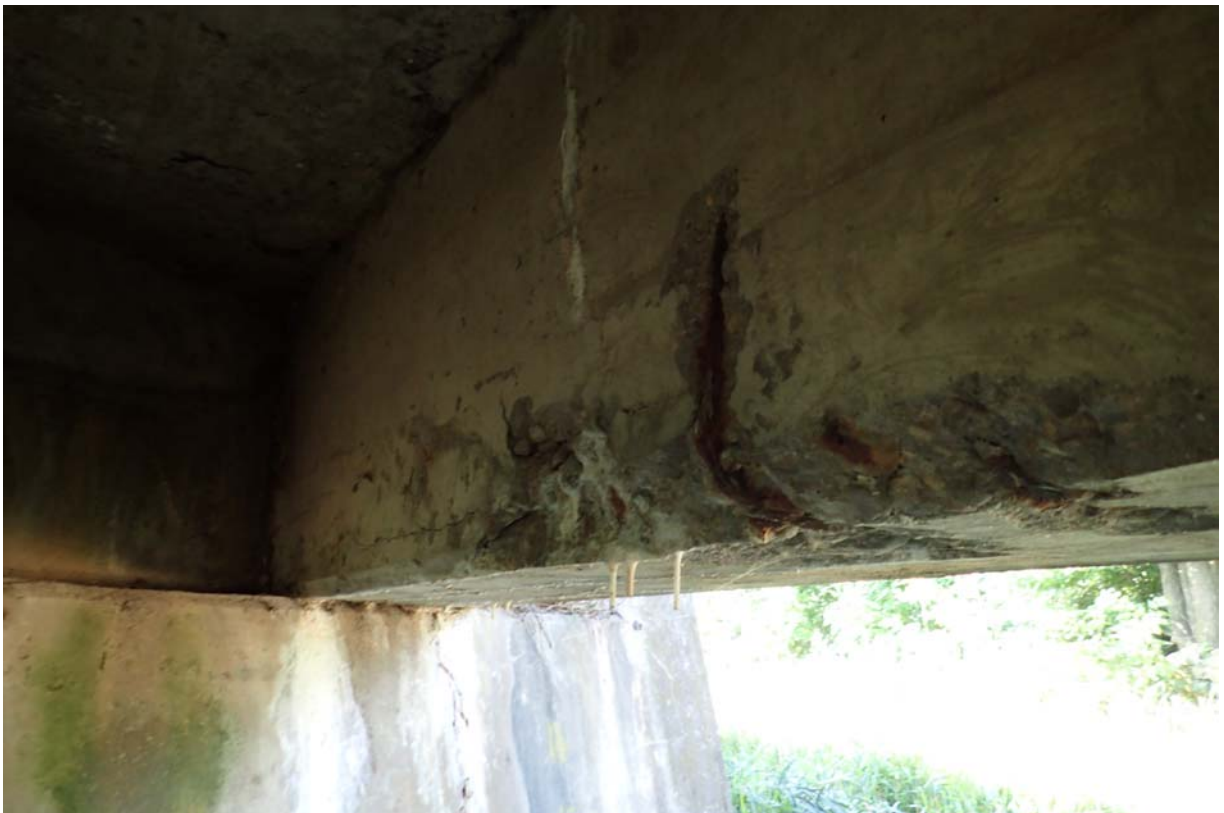
View of moderate cracking and spalling with exposed steel in the interior face of the upstream beam near abutment 2.
