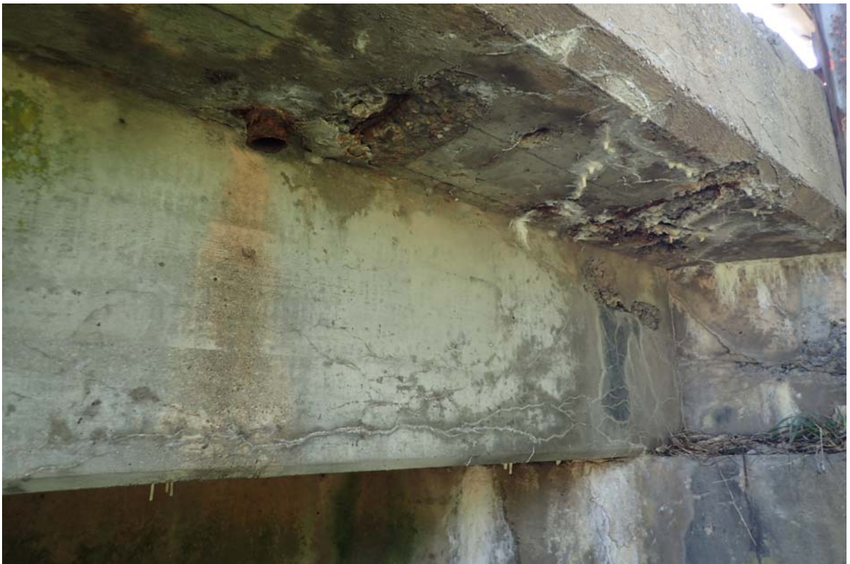
View of minor sized heavy intensity of cracking in the exterior face of the upstream beam and diaphragm at abutment 2. Notice the moderate to heavy spalling in the upstream deck overhang.
