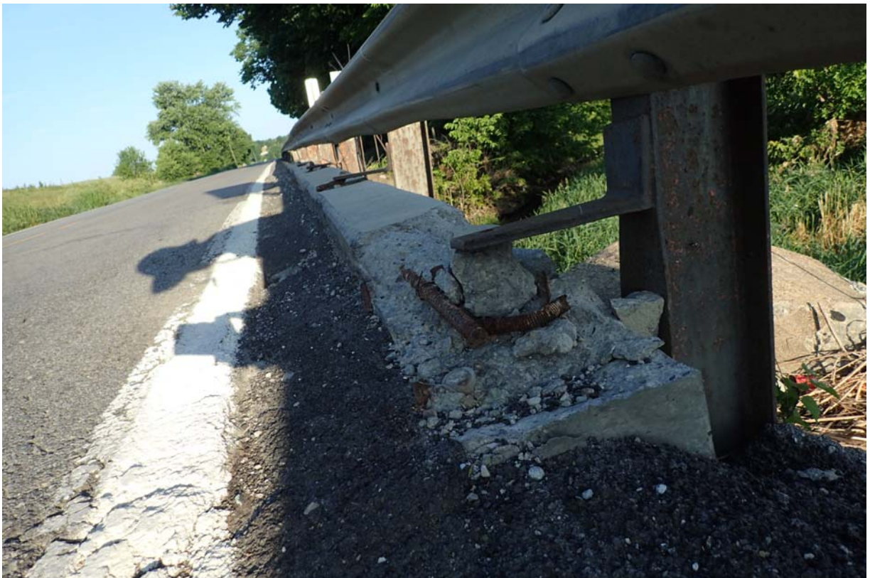
View of broken/spalled area in the downstream curb at abutment 2. Notice the guardrail post is no longer connected.
