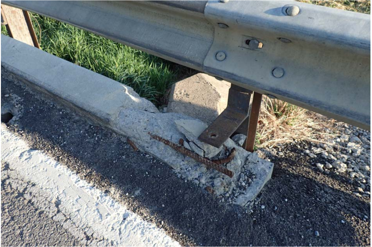
View of broken/spalled area in the downstream curb at abutment 2. Notice the guardrail post is no longer connected
