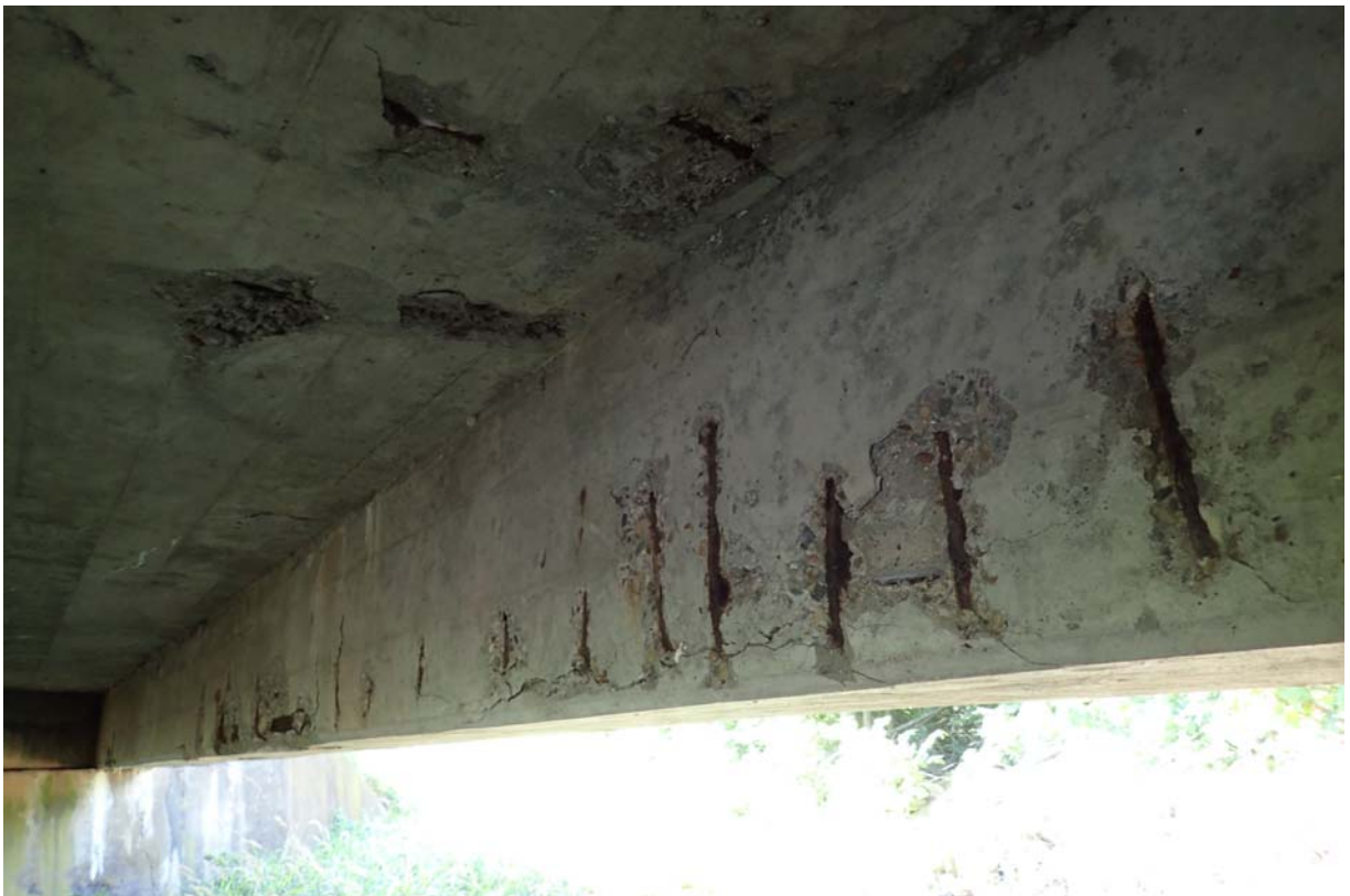
View of several small to medium sized spalls along the interior face of the upstream beam.
